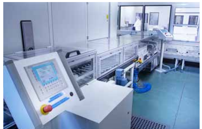
Industrial component cleaning unit with enclosed conveyor belt for the transport of ultra-fine cleaned goods into the clean room
